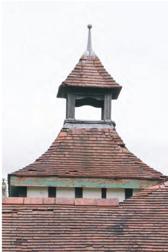
Plate 36. Detail of entrance tower roof of Sports Pavilion (Grade II Listed). Looking east.
