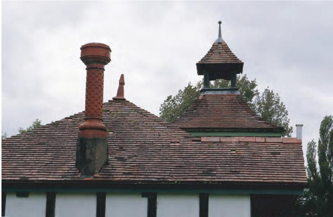
Plate 32. Roof and chimney detail of Sports Pavilion (Grade II Listed). Looking west.
