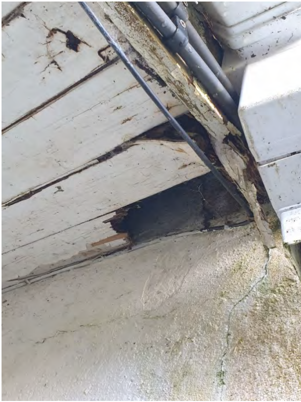
Hole in damaged wooden cladding on the underside of small roof connecting Building 1 and Building 2
