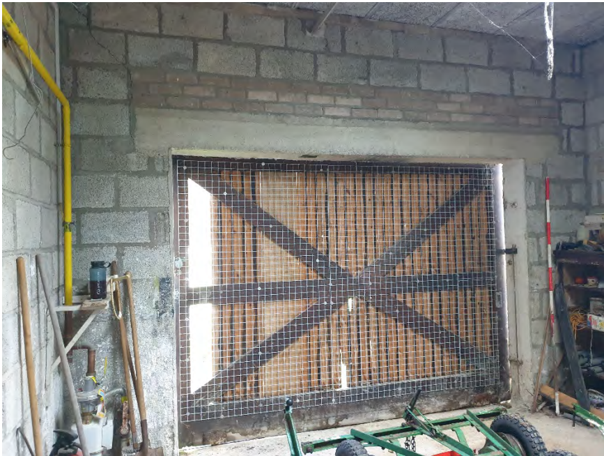
Damaged wooden sliding door on the western elevation creating access into the maintenance store
