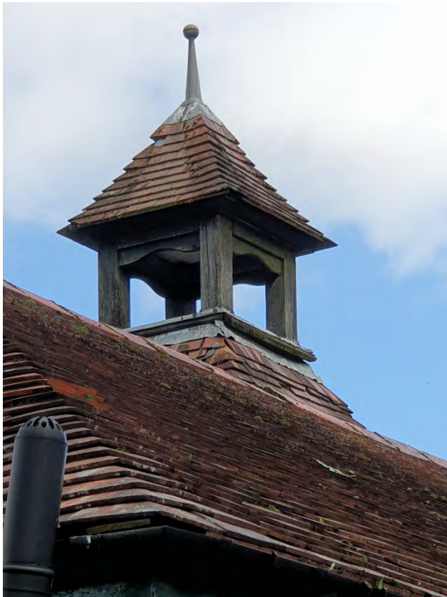
Gaps created by lifted, missing and damaged roofing tiles on bellcote
