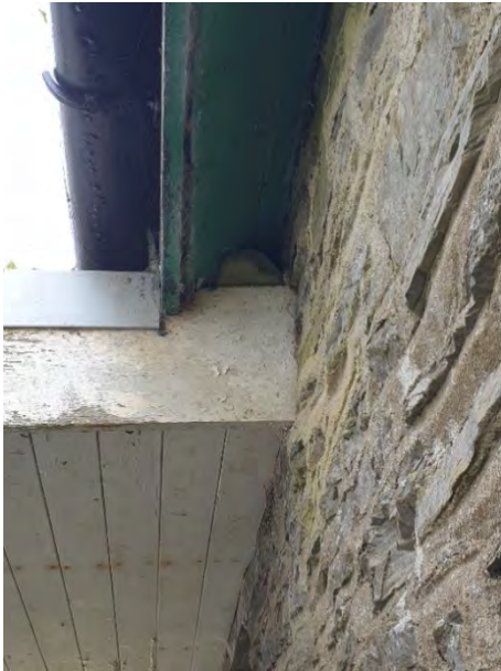
Gap into void between small roof connecting building with adjacent Changing Rooms Block to the south and angled soffit box
