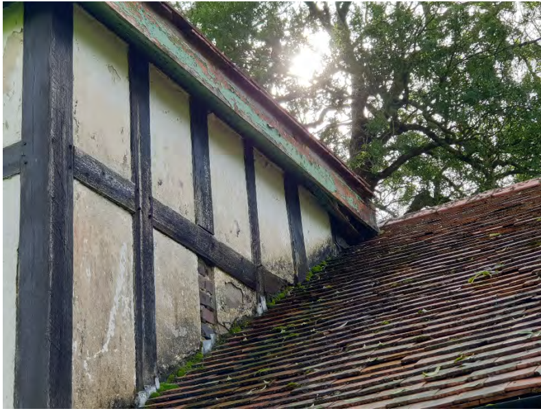
Gap created by damaged soffit box in the corner where central entrance block meets main roof
