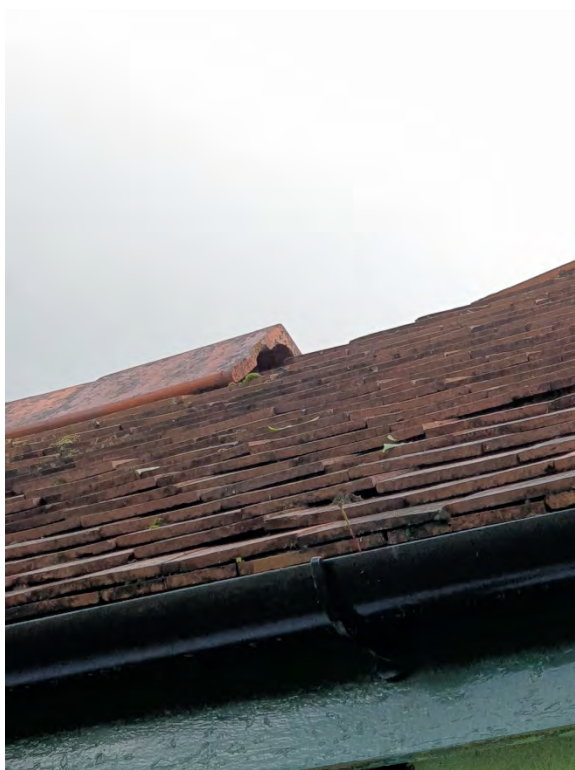
Gap at end of ridge tile and lifted roofing tiles
