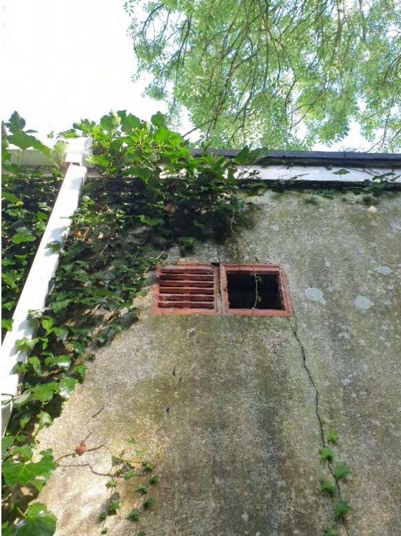
Damaged vent to the rear (southern elevation) – note - doesn't provide entrance into the interior of the building
