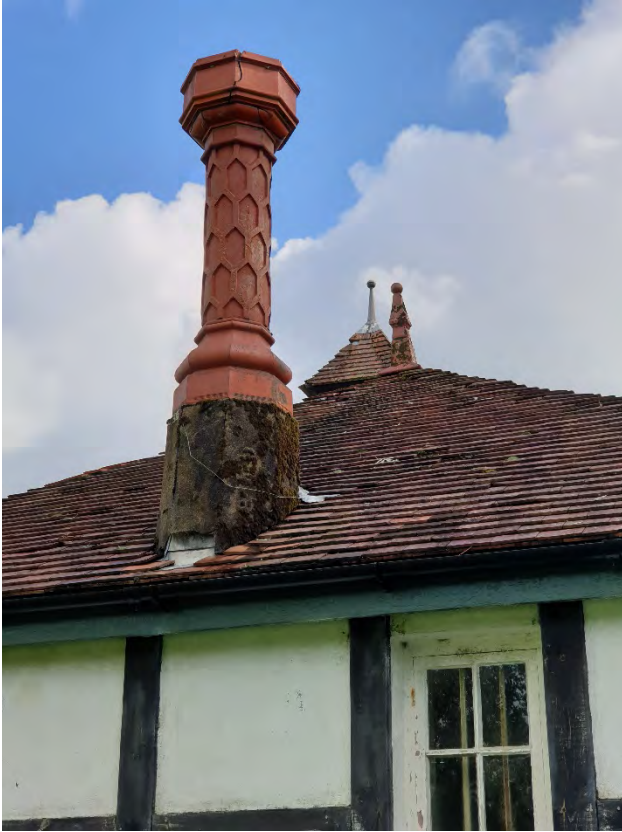
Lifted leaf flashing at base of moulded terracotta chimney and gaps created by lifted, missing and damaged roofing tiles
