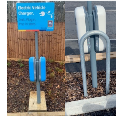
5 Aldi: EVCP post and dual chargers. Galvanised steel protection hoop
