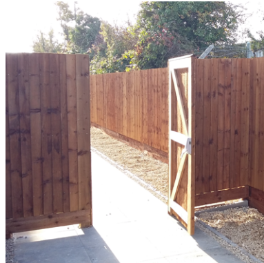
3 Close boarded fencing around car park and to rear of building, with integrated lockable gate with emergency push pad
