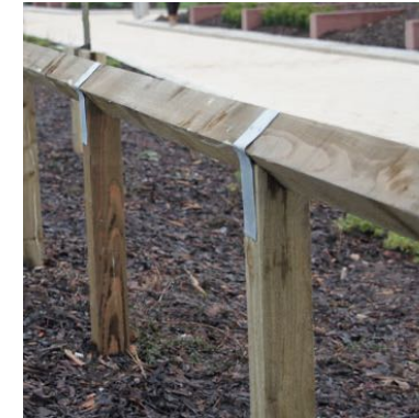
5 Timber Knee Rail with 100mm wide zinc straps. Located along perimeters of soft landscaping
